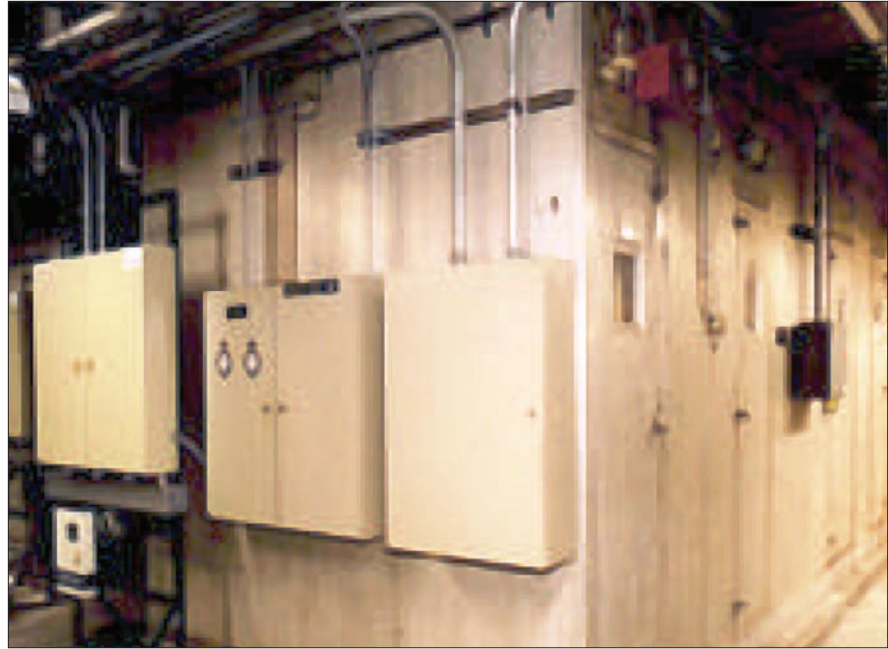
Figure 1: Air Handler Unit —Each AHU is designed to provide approximately 20,000 CFM of conditioned air to a space containing a volume of approximately 80,000 cubic feet, thus creating 15 air exchanges per hour or a fresh air turnover every four minutes.
